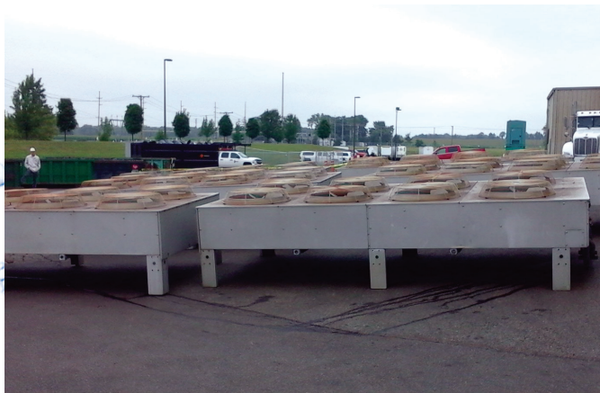
NIMBUS replaced these seven 8-fan dry air coolers with two 5-fan VIRGA III systems.
